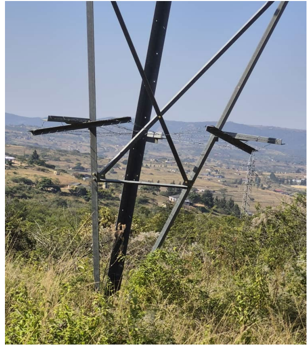
Collapsed vandalised 400 kV tower in Eswatini
