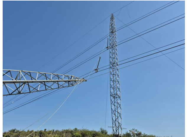
Collapsed vandalised 400 kV tower in Eswatini
